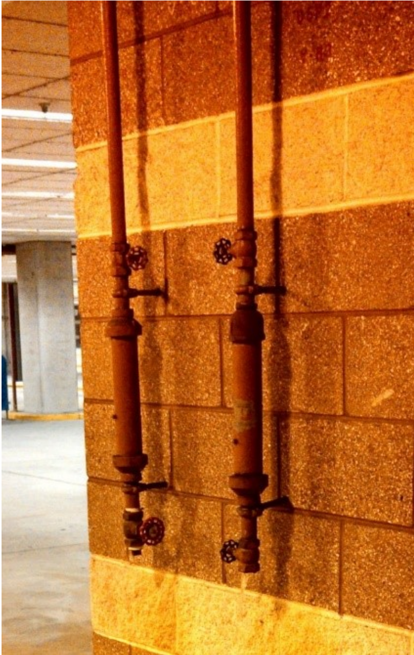
Example Drum Drips (Auxiliary Drains) in a Parking Garage.
